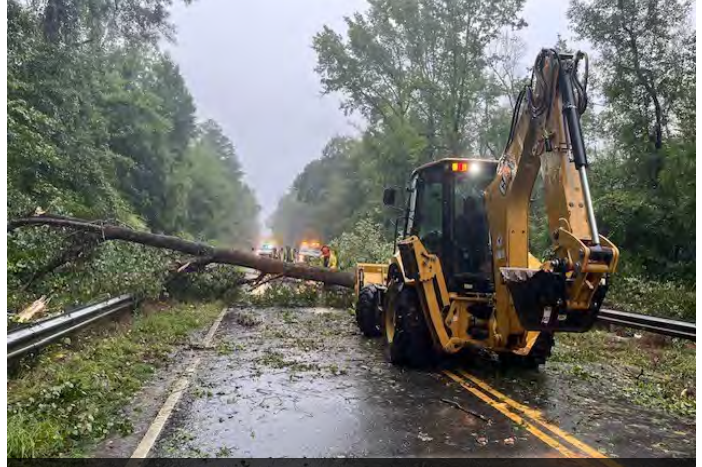
SRNS Site Services clears a fallen tree out of an SRS roadway during Hurricane Debby.
